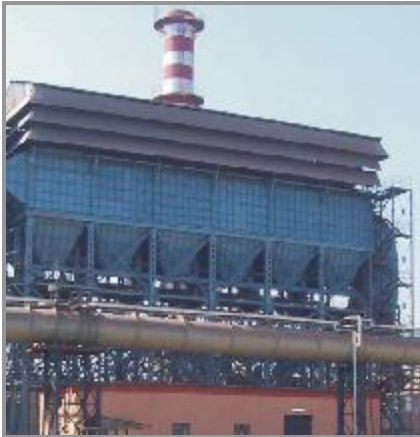
Specialised Dedusting system in a cast house
