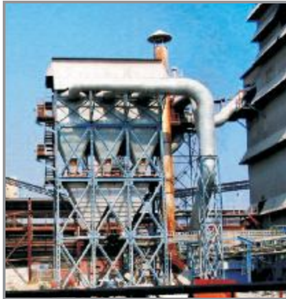
Modular pulse jet bag filter on a lime / dolomite kiln
